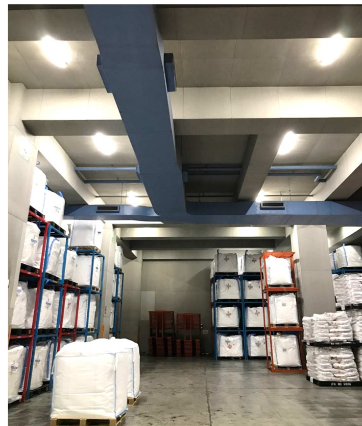
Ohi warehouse wholly replaced with LED bulbs
